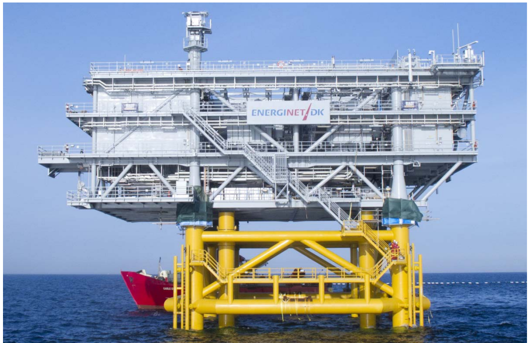
Transformerplatform – Anholt Havmøllepark
